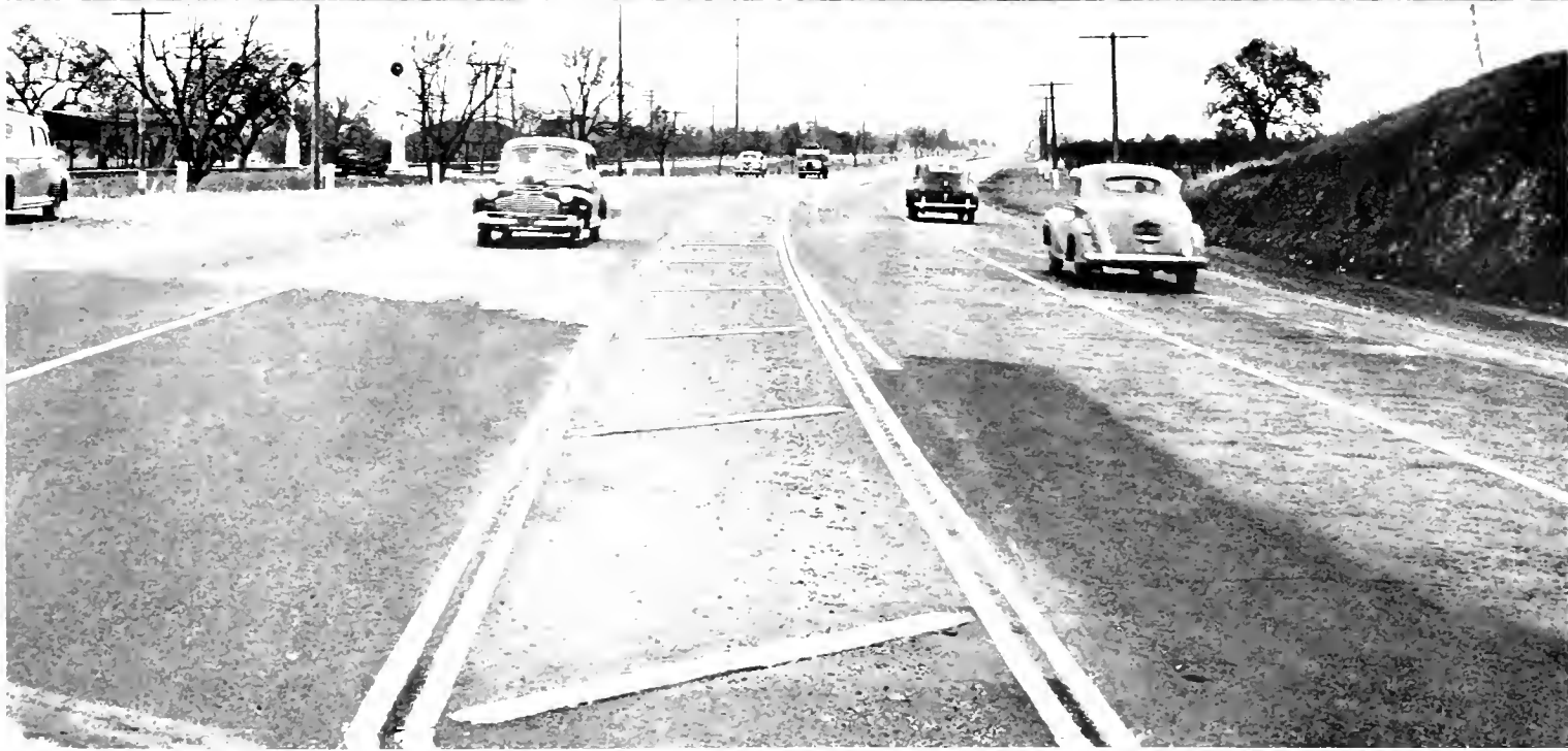
These photographs show types of divided highway construction on new improvement on U. S. 101, north of Gilroy
